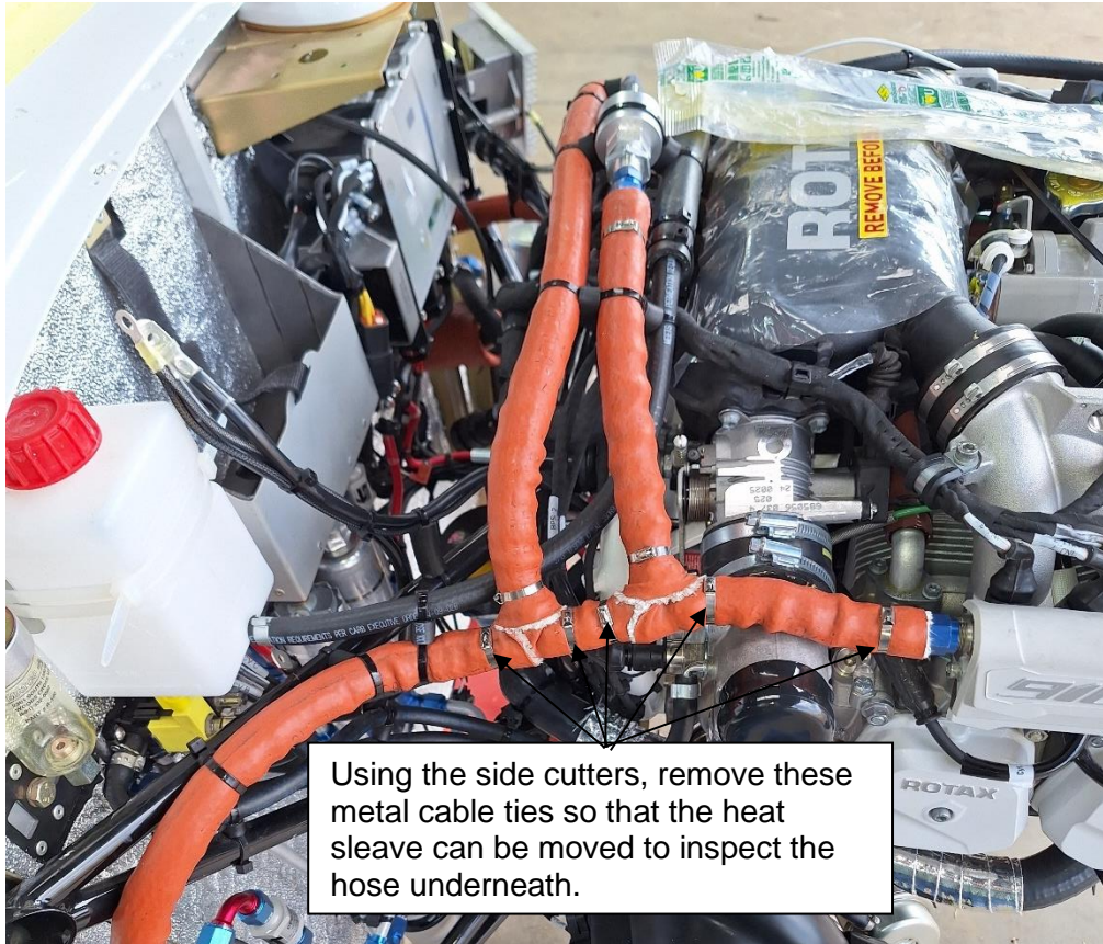
Figure 10: Example of cable ties to be removed.
